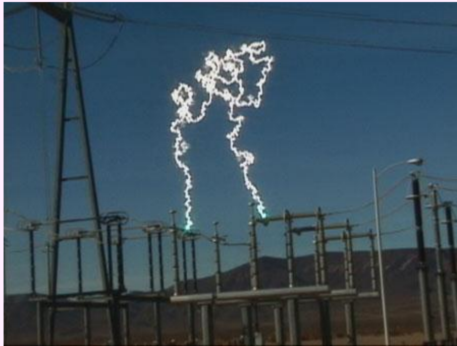
See: Electrical Overload
